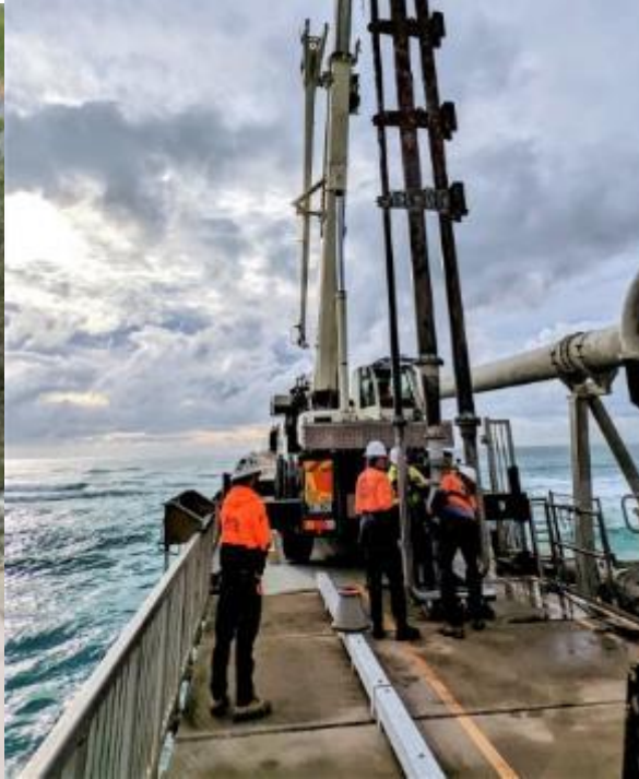
SBS Guide Rails project
